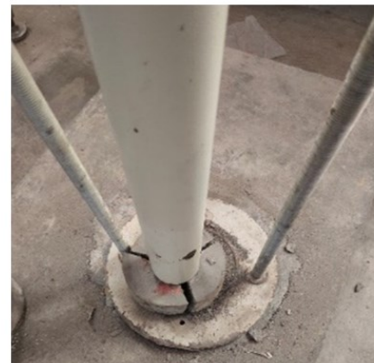
(a) Failure mode
