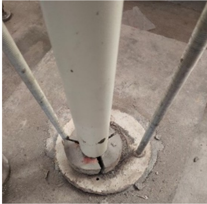
(a) Failure mode
