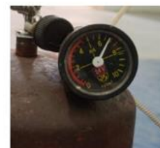
Figure 4. H 2 storage tank
