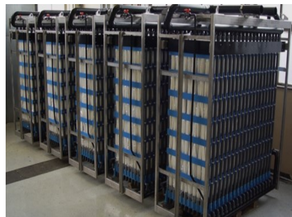
Figure 2. View of MBR Membranes
