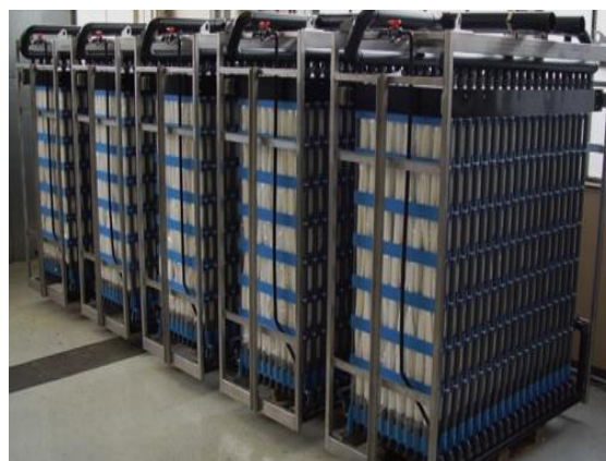
Figure 2. View of MBR Membranes
