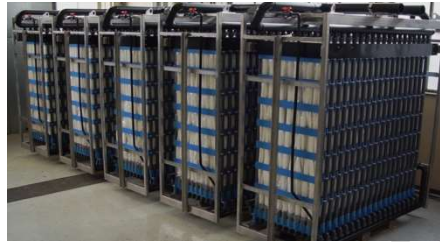
163 164 Figure 2. View of MBR Membranes
