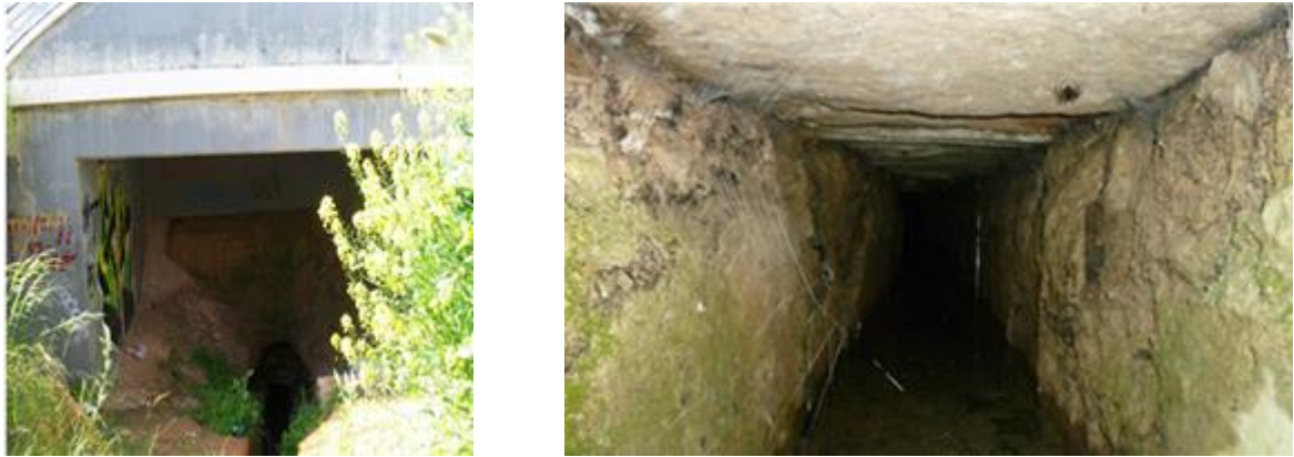
Figure 9. The end of the surface branch and the start of the underground main branch towards the Olympic village (a), and the inside of the underground canal (b)
